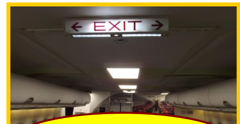
Illuminated EXIT sign controlled by the FAP
