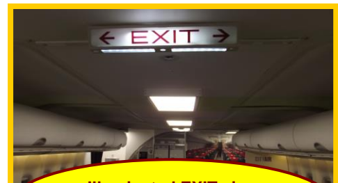
Illuminated EXIT sign controlled by the FAP
