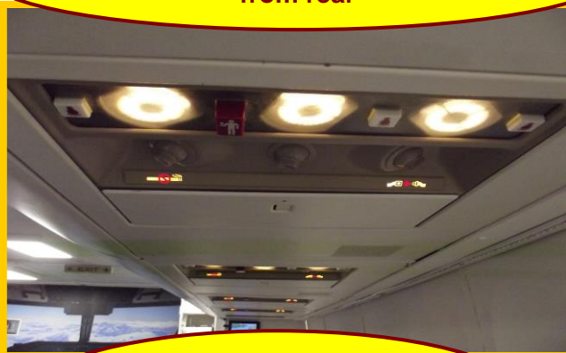
Fully operational Passenger Service Units – controlled by the FAP
